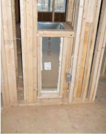
Duct chase between floors.
