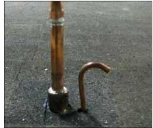
Figure 1-38 – Copper top hat flashing with gooseneck for sensor wire. In this example, the flashing sheet was installed entirely under a course of shingles. If the flashing falls on a seam or has inadequate coverage by the upper course, this is necessary.
