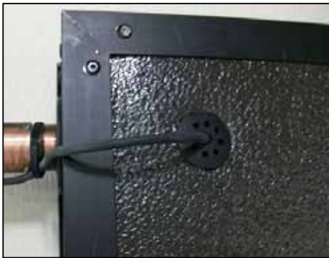
Figure 1-22 – Sensor probe installed on absorber plate through collector vent
