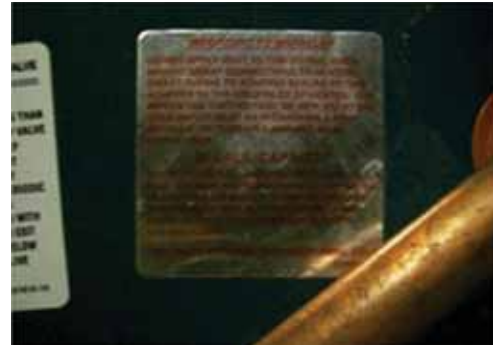
Figure 3-3 – Example of tank label with pressure rating
