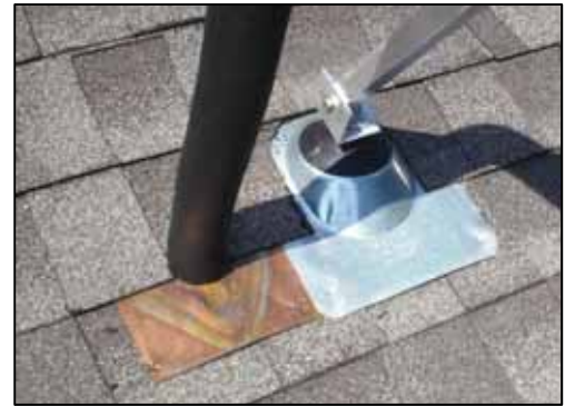
Figure 1-35 – Roof boot (on right) used to seal cylindrical standoff (copper top hat pipe flashing on left)
