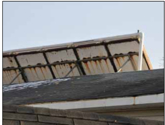
Figure 1-29 – Galvanic corrosion on a collector array due to direct contact of dissimilar metals between the collectors and racking
