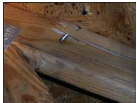
Figure 1-32 – Improperly installed lag bolt (image courtesy of Mark Thornbloom)
