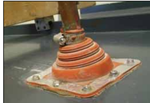
Figure 1-39 – Silicone pipe flashing on metal roof. Note that the sealant between the flashing and the roof should extend beyond the flange for inspection purposes. Also, care should be taken to avoid squeezing the silicone through the hose clamp, as it is here.
