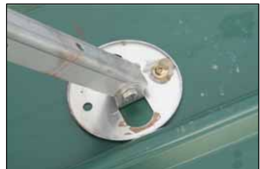
Figure 1-34 - Example of improper attachment of tilt rack foot. Without a bolt in the front hole, live loads would pry the foot from the roof surface. A neoprene gasket should also be installed between the foot and metal roofing to provide a durable seal for the bolt penetration and to isolate dissimilar metals.
