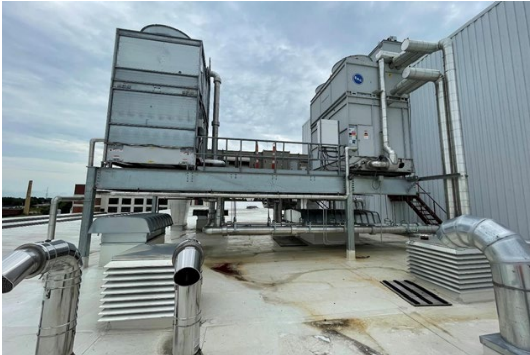
Figure 4. Typical Cooling Tower
