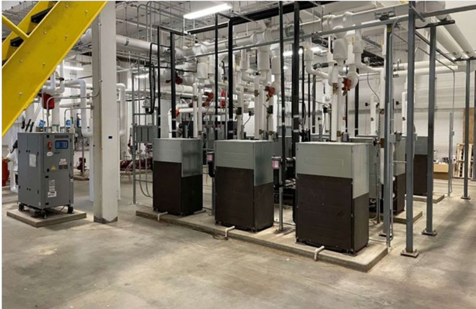
Figure 6. Typical Boiler Room
