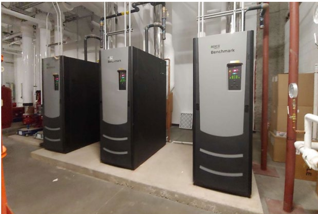
Figure A-1. Hot Water Boilers at Northland
