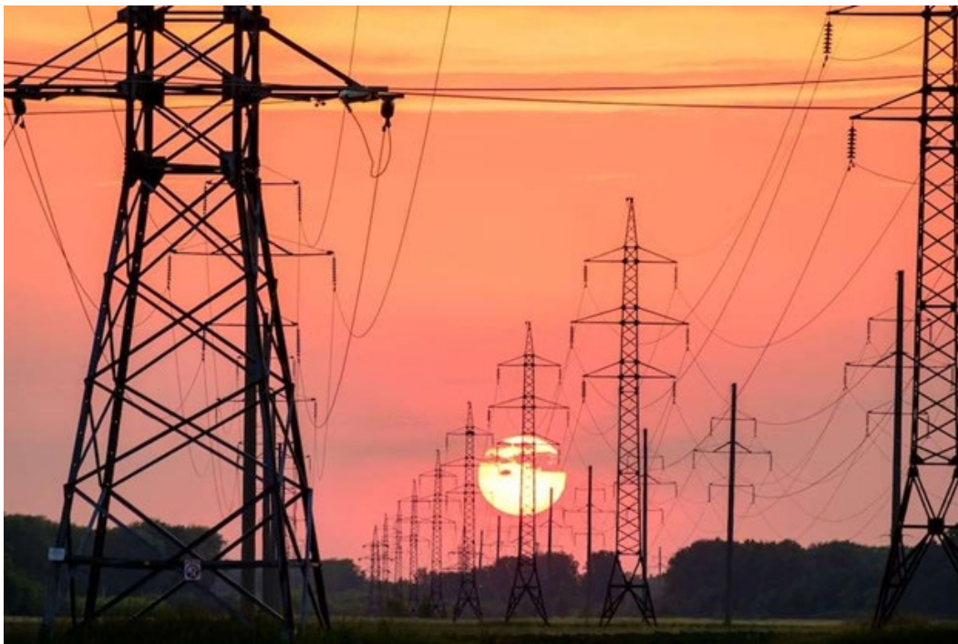
Figure 5. Typical High Voltage Transmission Lines
