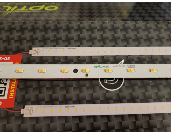
DEC installed magnetic LED retrofit strips at a number of their facilities. These provide a low-cost way to decrease energy use for lighting. Credit: DEC
