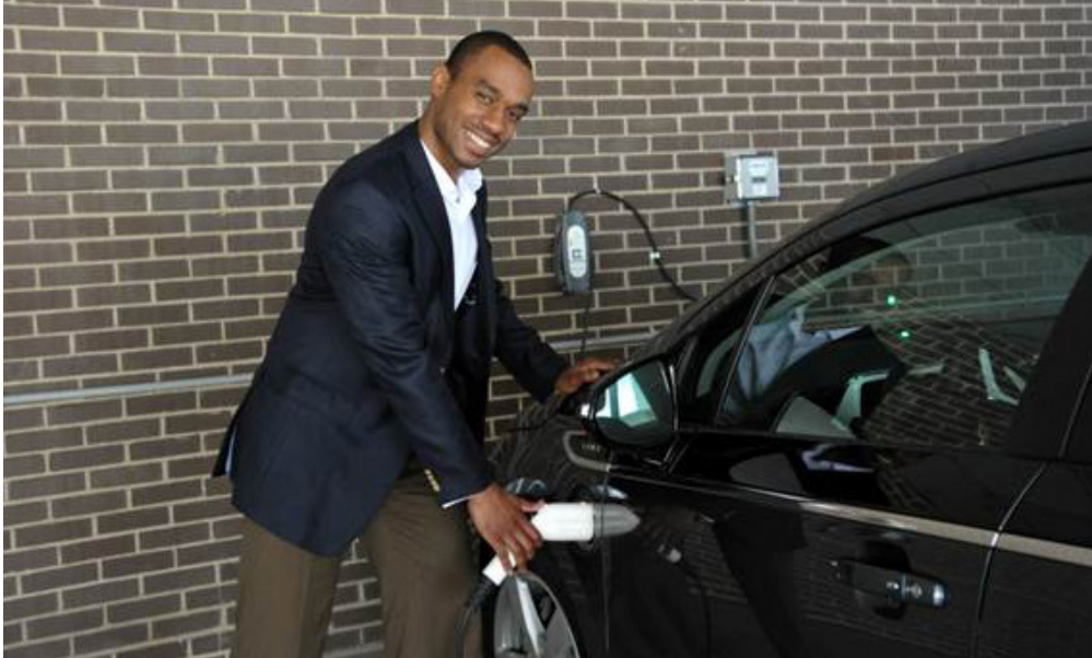
NYPA employees can charge their EVs at work using Level 1 charging stations. Photo credit: NYPA
