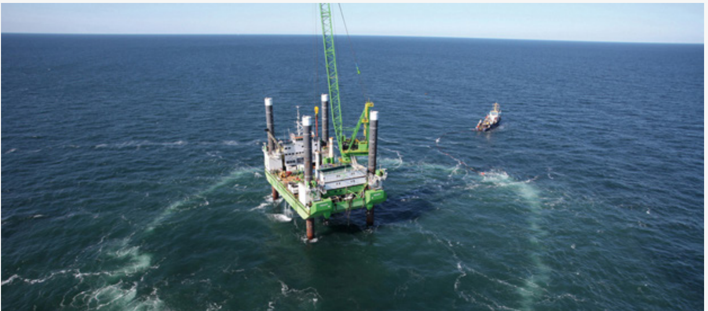
Bubble curtain being used to mitigate sound levels from pile driving during construction of a wind farm in Germany in 2012. Credit: Trianel GmbH
