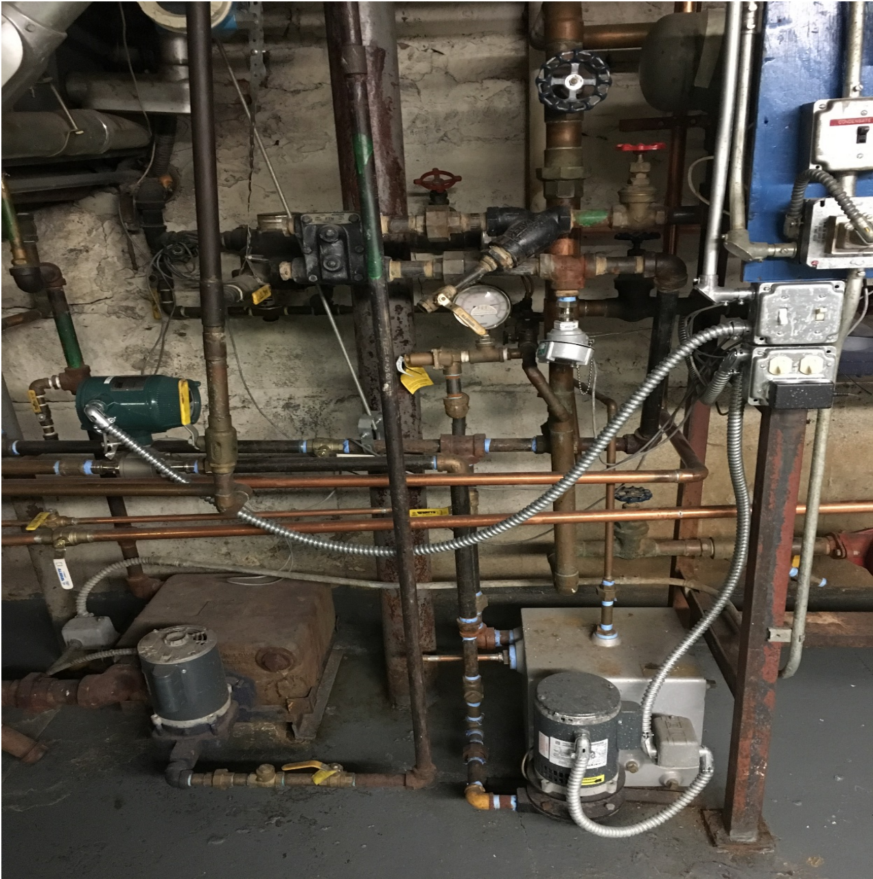
Figure 16. Condensate Tank, Condensate Pump, and Control Panel
