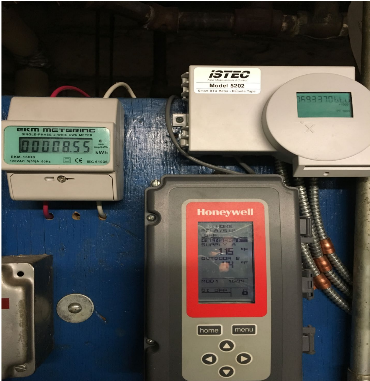
Figure 17. Electric Meter (EKT Metering), ESTEC BTU Meter, and Honeywell Temperature Display
