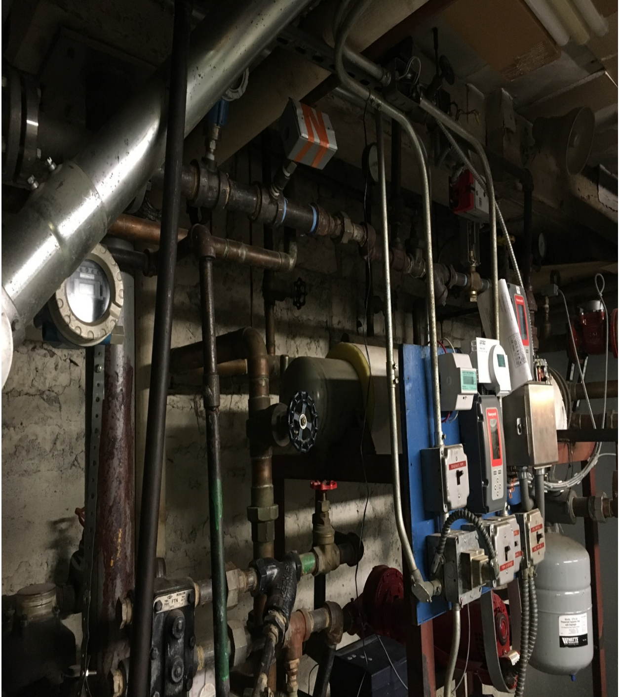
Figure 9. Tube-and-Shell Heat Exchanger, Control Panel, and the Expansion Tank
