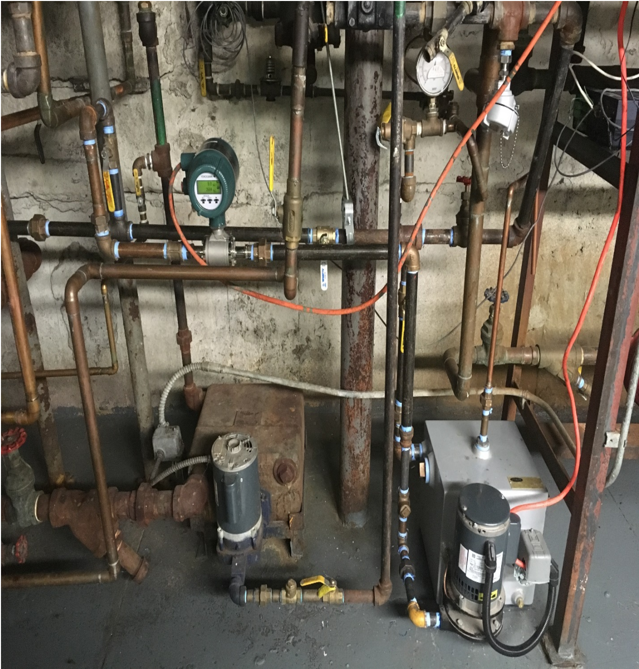
Figure 13. Condensate Tank, Condensate Pump, and the Condensate Flow Meter
