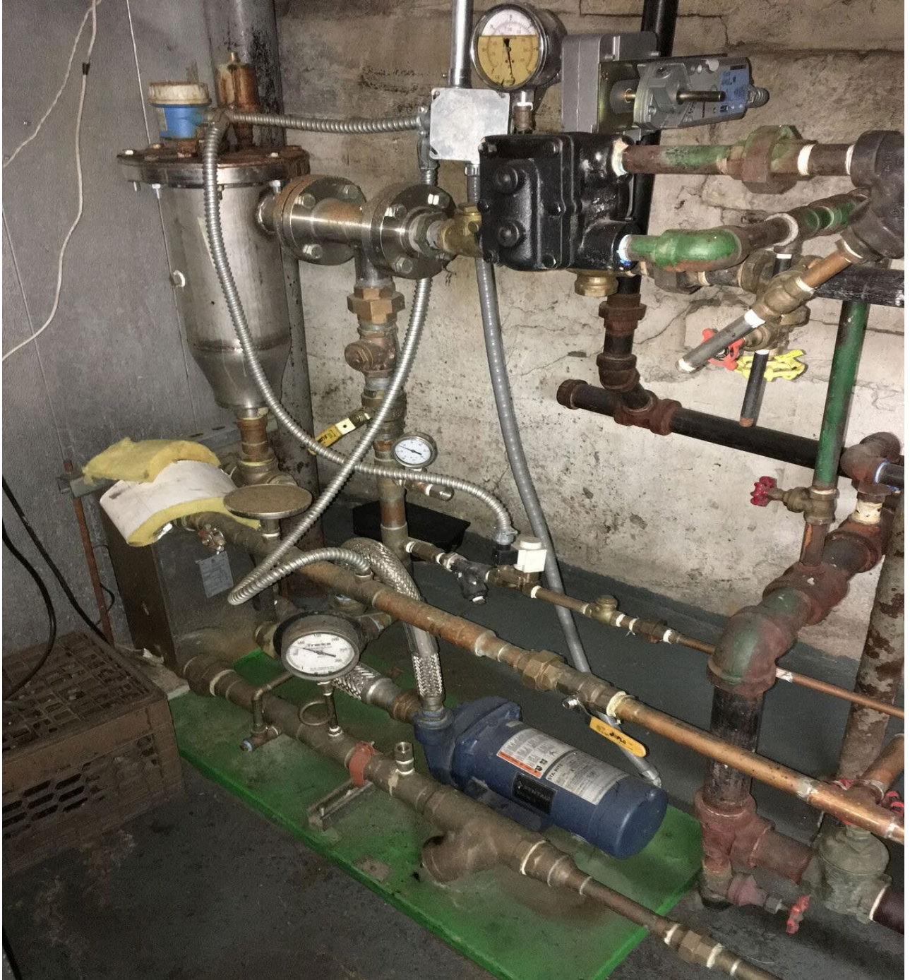
Figure 12. Fisonic Device, Vortex Tank, Plate and Frame Heat Exchanger, and Water Circulating Pump
