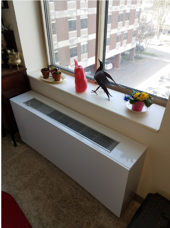
Photo 2. Nonstandard size PTAC with hot water coil
