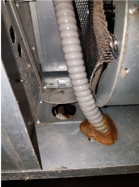
Photo 3. Passive make-up air vent in PTAC
