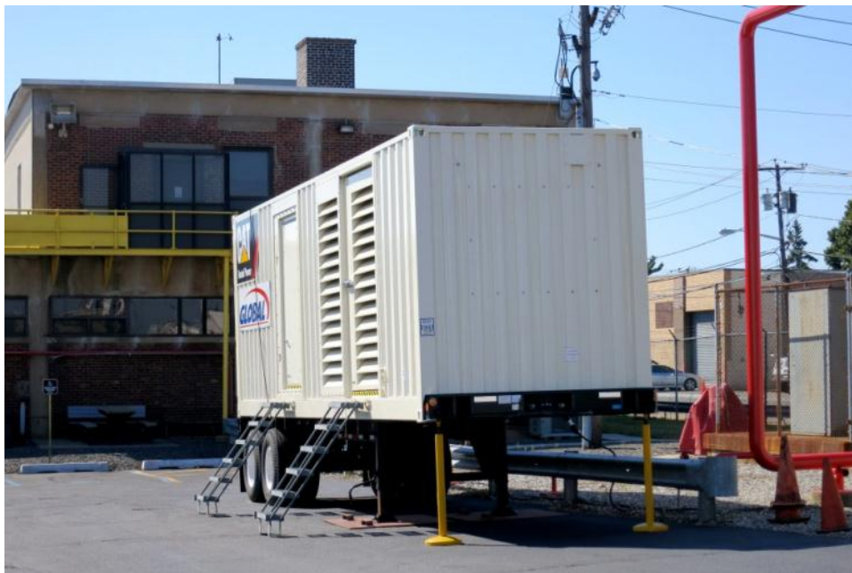
Figure 31. Mobile, Trailer-Mounted Diesel Backup Generator
