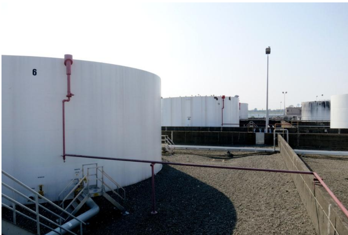
Figure 24. Tanks Are Filled with Product or Water to Prevent Tank Movement During Flooding
