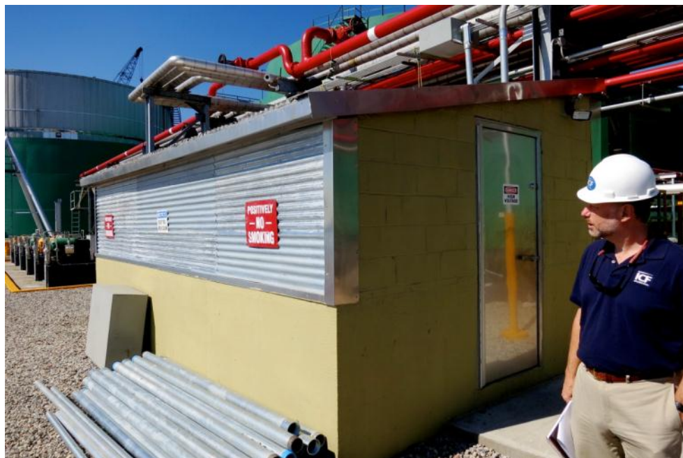
Figure 27. Motor Control Center Hardened Against Flooding
