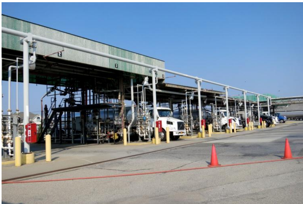
Figure 5. Truck Loading Rack
