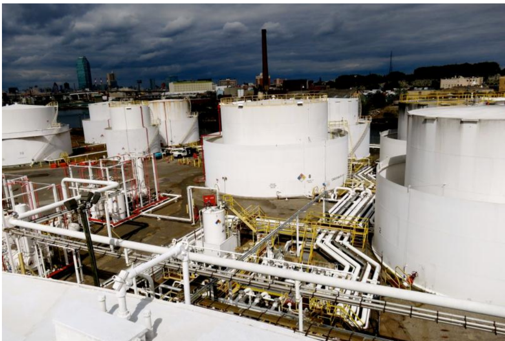
Figure 2. Tank Farm with Ringwalls Around Tanks
