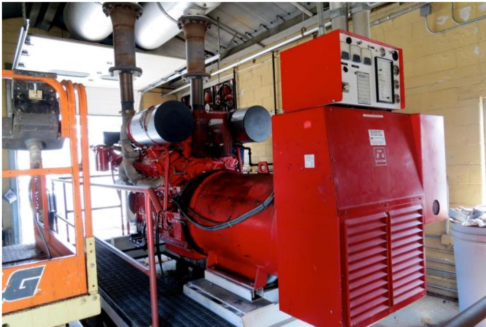
Figure 30. Fixed Diesel Backup Generator
