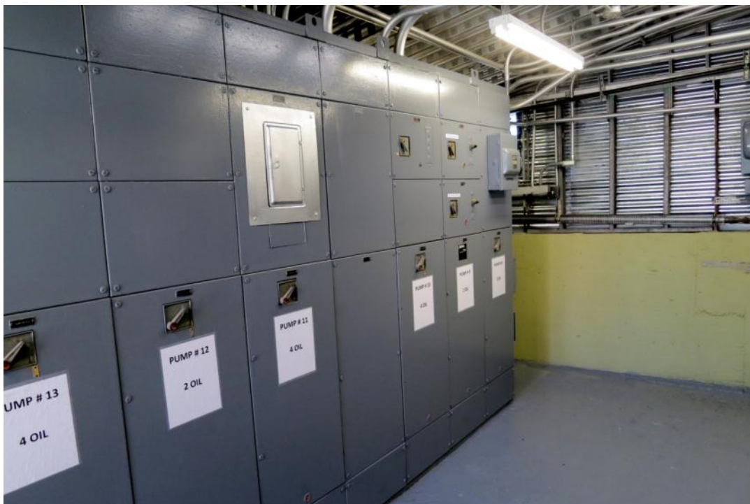
Figure 7. Motor Control Center
