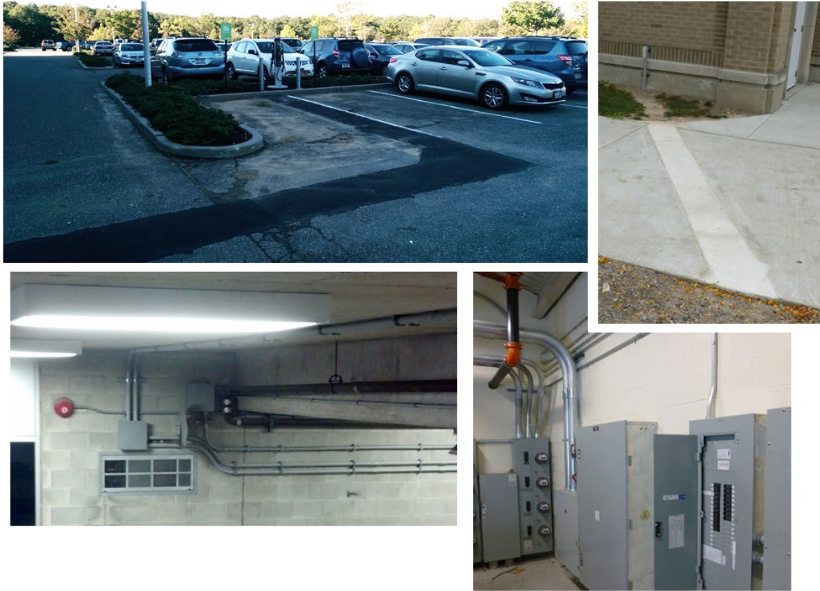
Figure 8. Example EVSE Installation Factors
