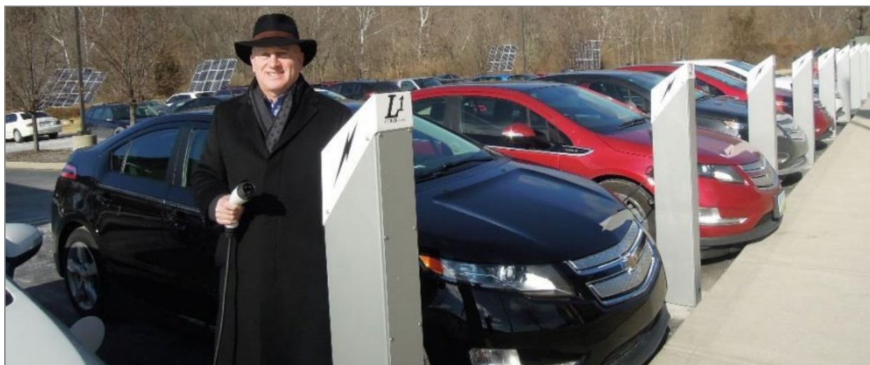
Figure 6. Example AC Level 1 EVSE Installation
