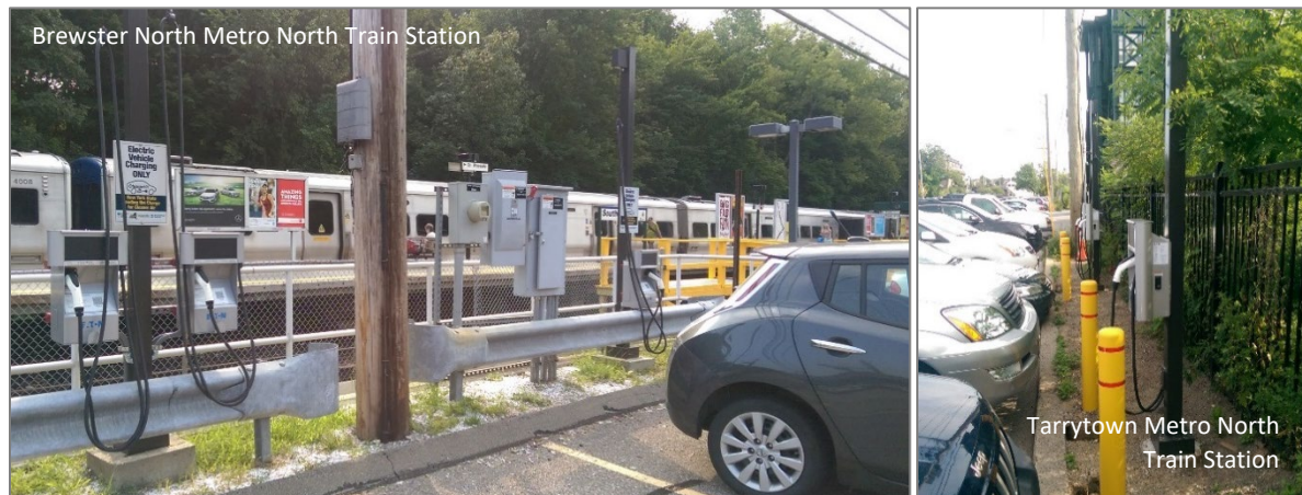
Figure 34. Example EV Charging Stations at Transit Locations
