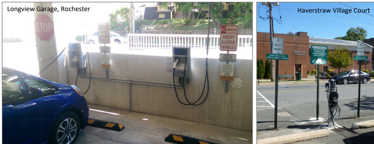
Figure 30. EV Charging in Multiuse Parking Lots and Garages Outside of NYC
