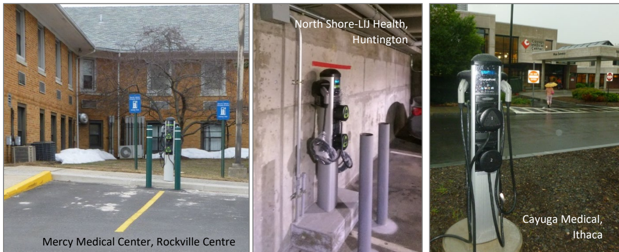
Figure 46. Example EV Charging Stations at Healthcare and Medical Facilities
