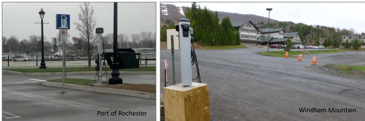
Figure 22. Example EV Charging Station Installations at Recreational Locations
