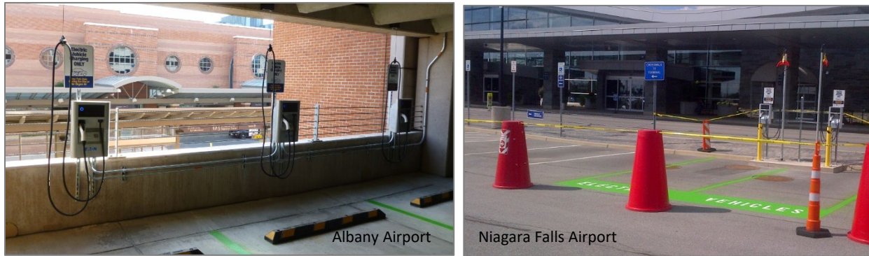
Figure 38. Example EV Charging Stations at Airports
