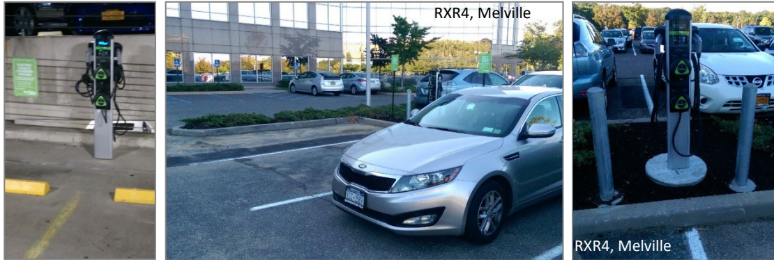
Figure 50. Example EV Charging Stations at Business Offices
