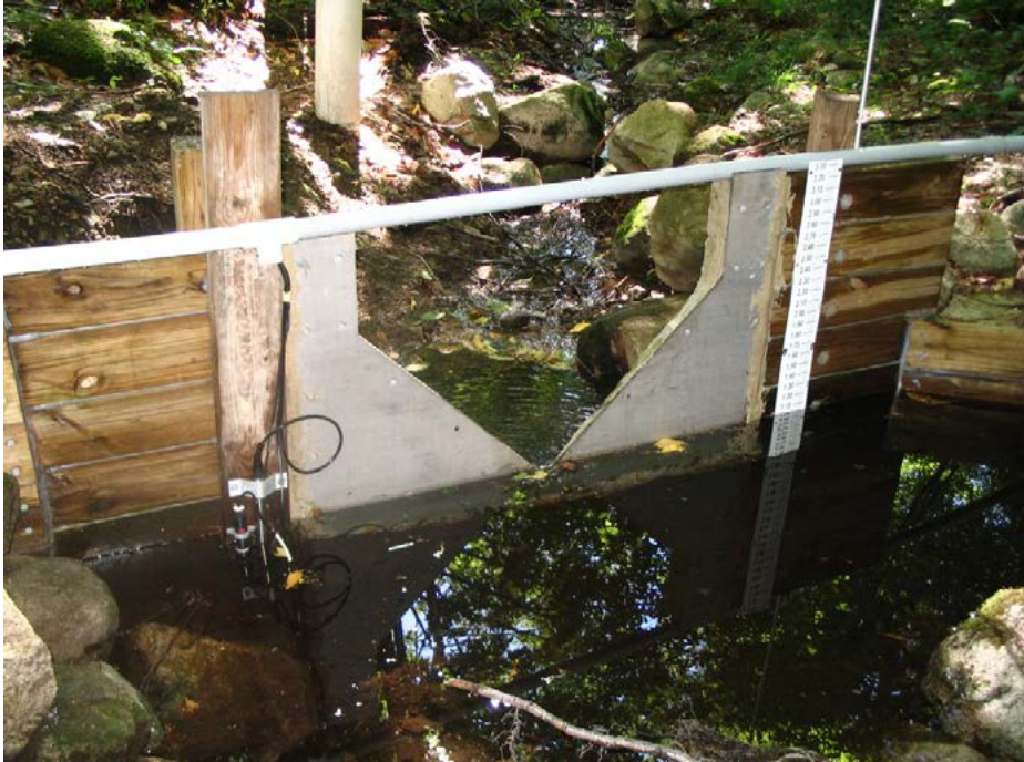
V-notch weir at sub-catchment 14
