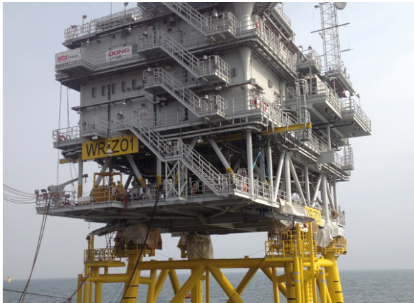
Figure 13. Westermost Rough Wind Farm Substation in Yorkshire, UK
