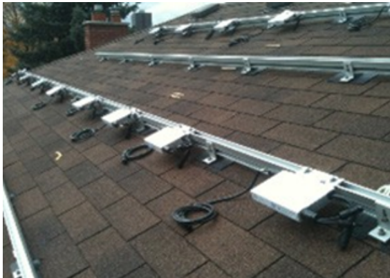
A Solar Electric Racking System
