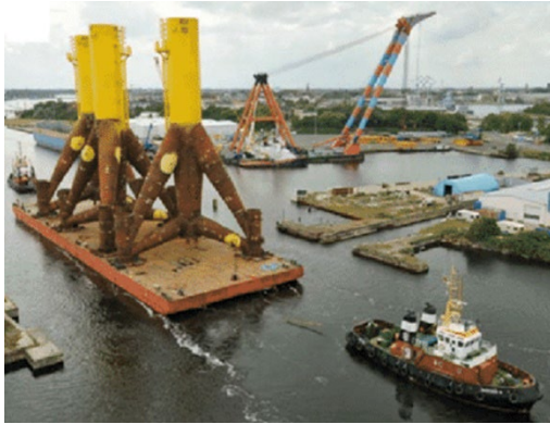
Figure 11. Installed on Site by a Barge-Crane Used for the Alpha Ventus Windfarm
