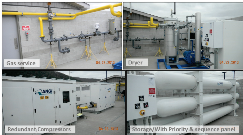
Figure 17. Fast-fill CNG Station Equipment (shown for a Cascade Configuration)
