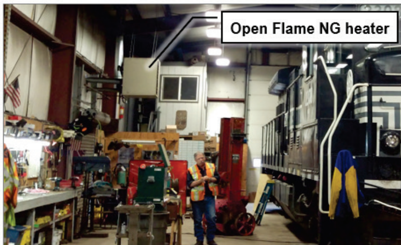
Figure 21. Existing Heating System
