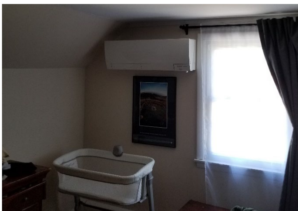
Master Bedroom Indoor Unit
