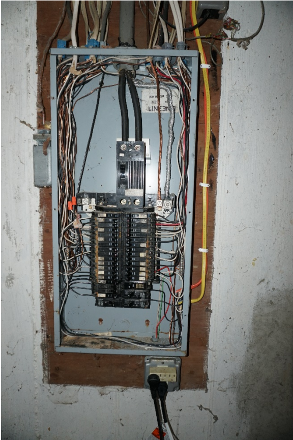
Electrical Panel Upon Arrival
