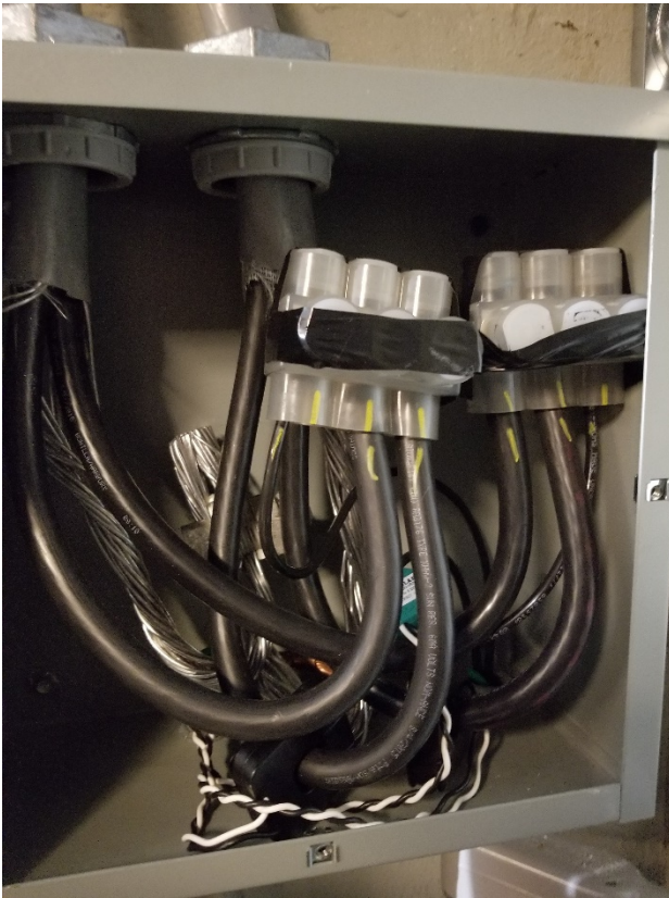
Mains Junction Box with Solar
