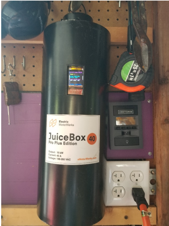
Level 2 EV Charger Located in the Garage
