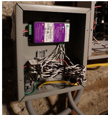
eGauge monitoring box
