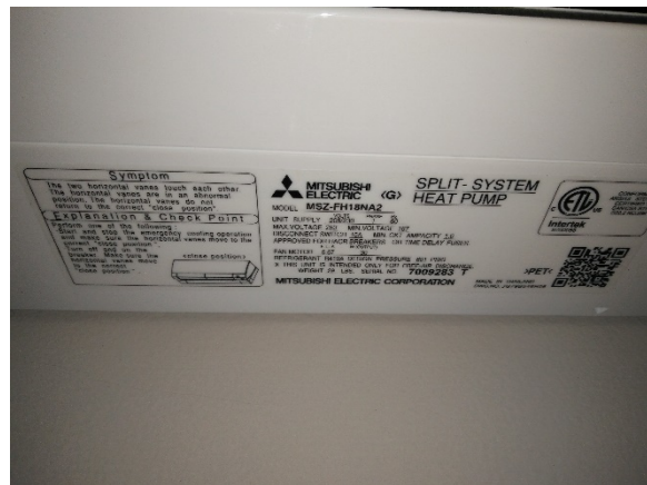
Indoor Unit Nameplate
