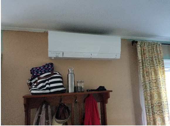
Kitchen/Dining Area Indoor Unit
