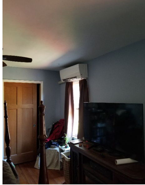
Master Bedroom Indoor Unit
