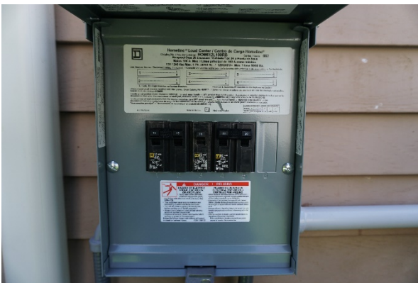
Separate Breaker Box/Subpanel by Outdoor Units
