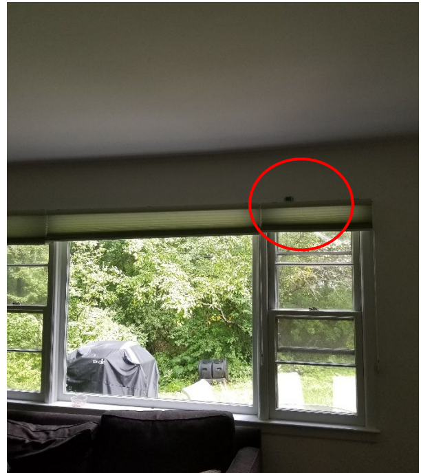
Temperature Data Logger in Family Room
