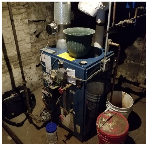
Natural Gas Boiler
