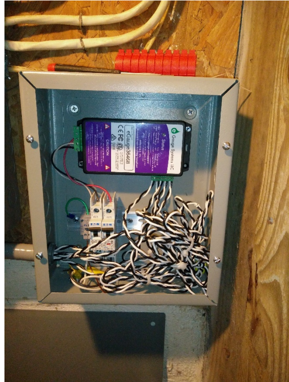
eGauge monitoring box
