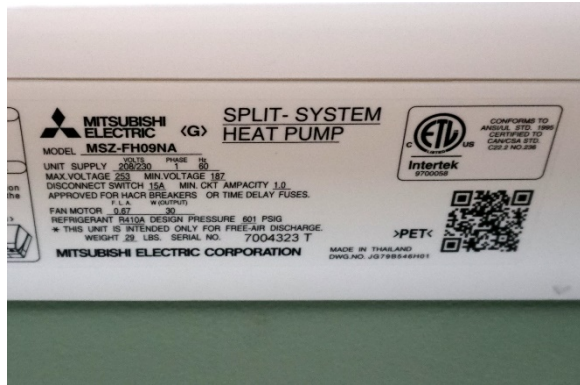
Master Bedroom Indoor Unit Nameplate
