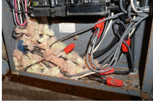
Exposed Wires Under Insulation Nest
