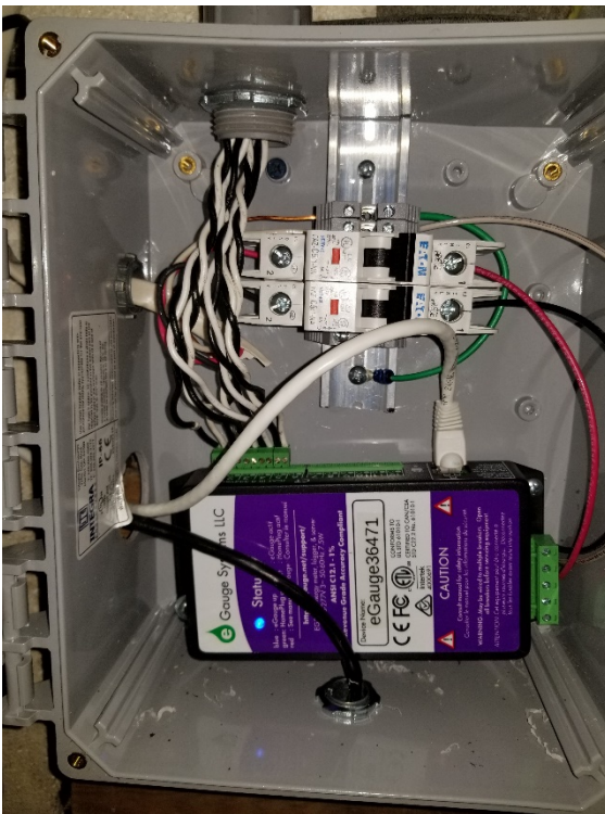
Data Logger Enclosure with eGauge
