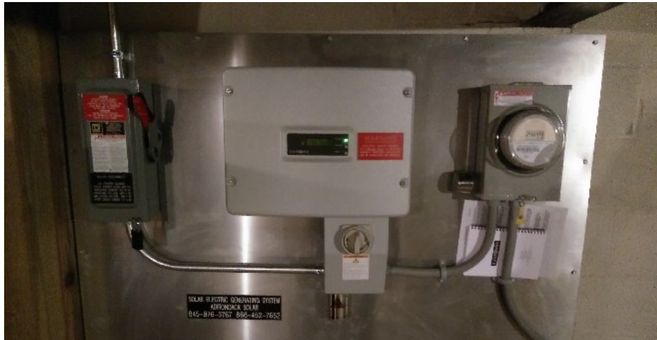
Solar inverter and generation meter
