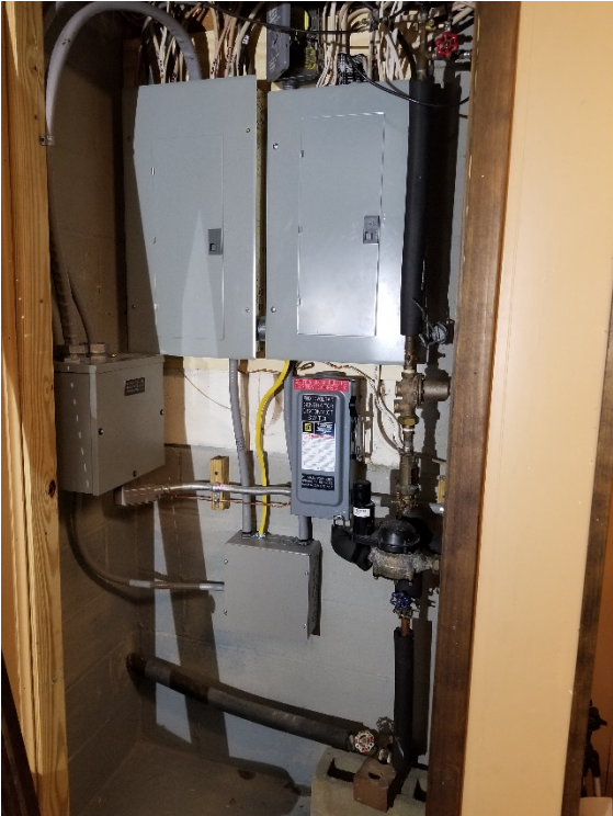
Main Electrical Panels with eGauge
