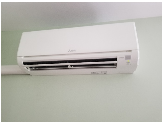
Office Indoor Unit
