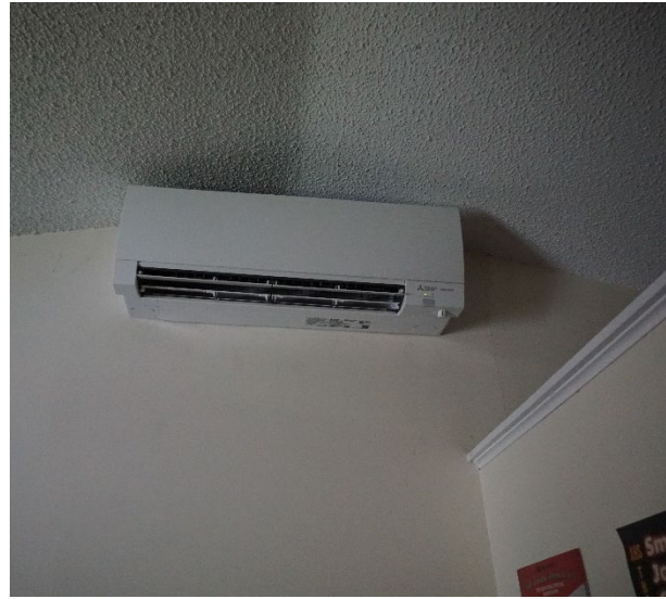
Living Room Indoor Unit
