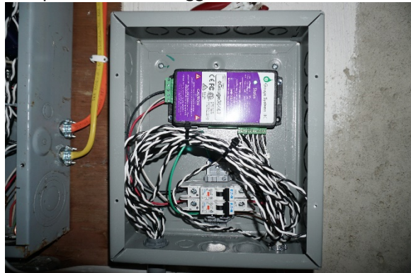
eGauge monitoring box
