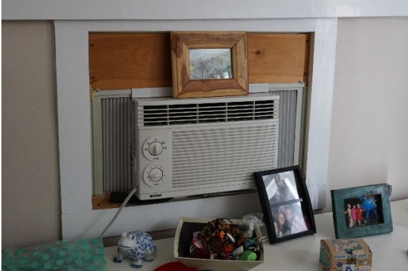
Window Air Conditioner, Master Bedroom
