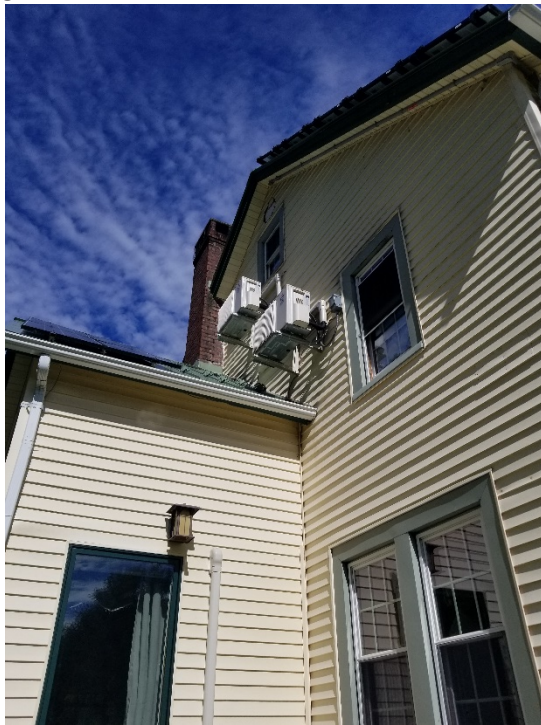
Two Old Outdoor Units and PV Array
