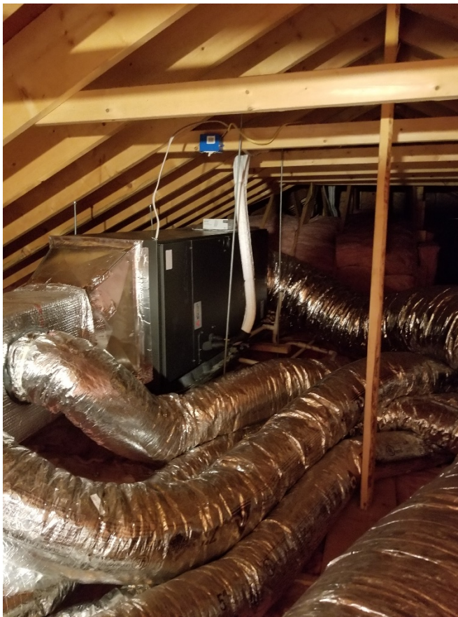
Air Handler Located in Attic
