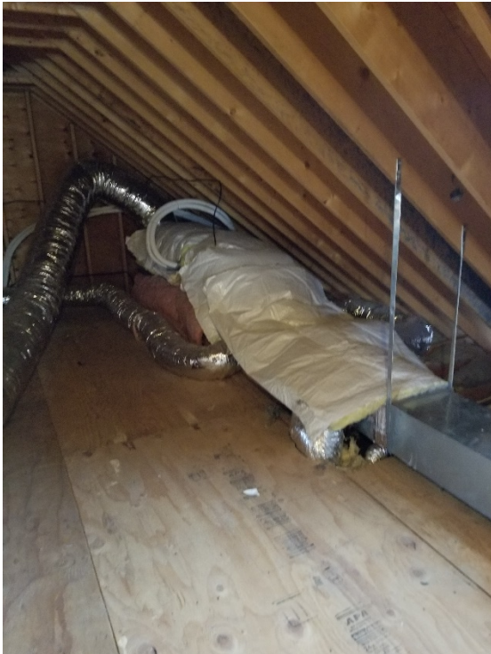
Air Handler Located in Attic
