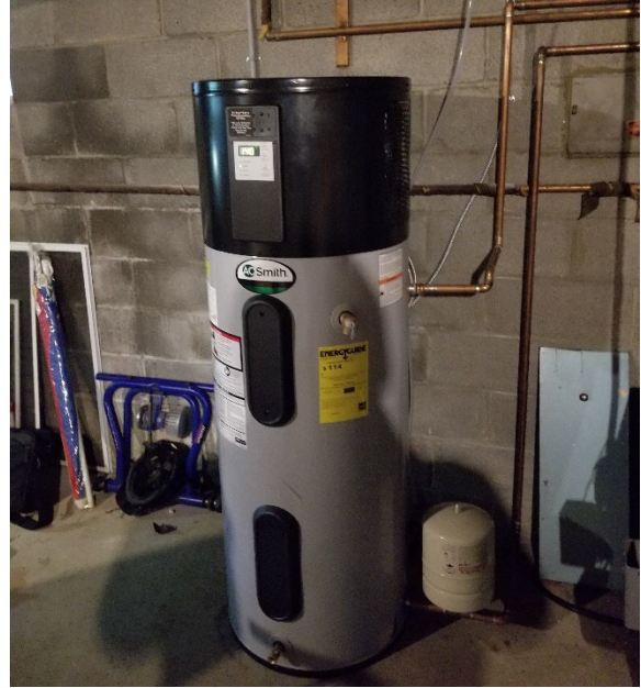
Electric Heat Pump DHW Tank
