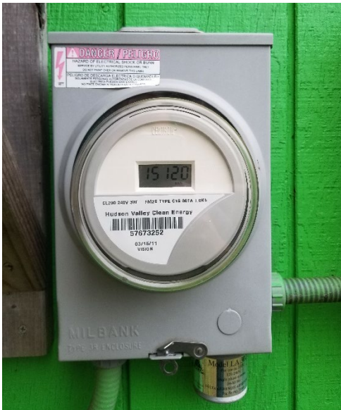
Utility Clean Energy Meter Located on Garage
