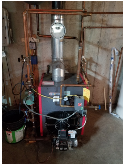
Fuel Oil Boiler
