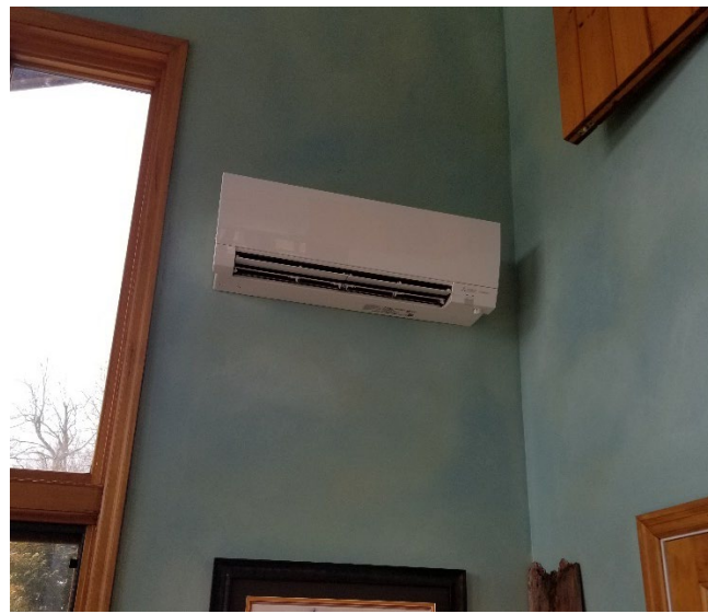
One of two Indoor Sections in Living Room
