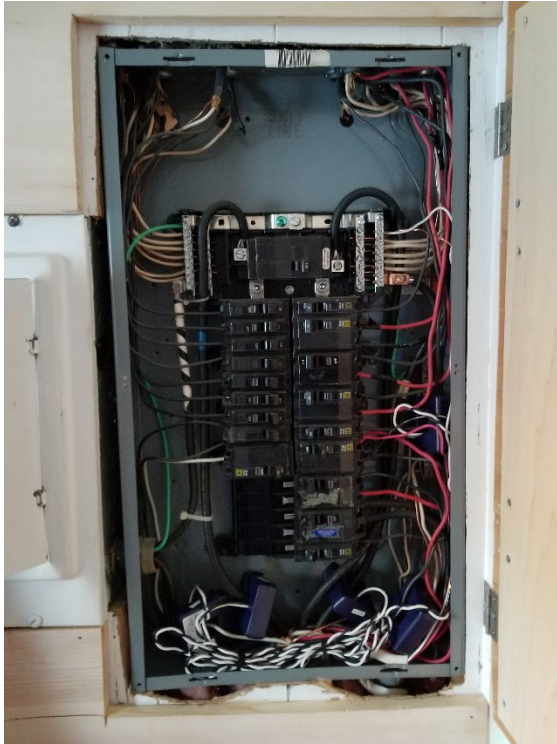
Main Electrical Panel with CTs
