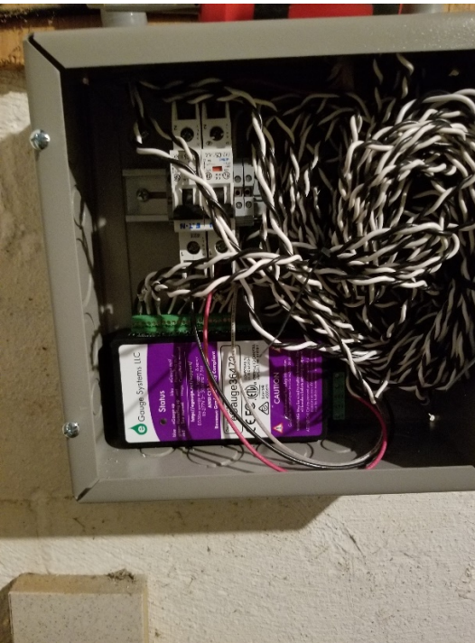
Data Logger Enclosure with eGauge
