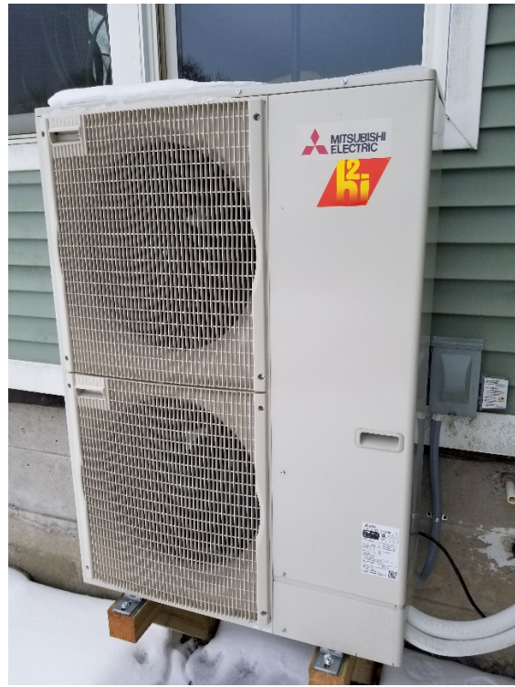
One of Two Outdoor Units
