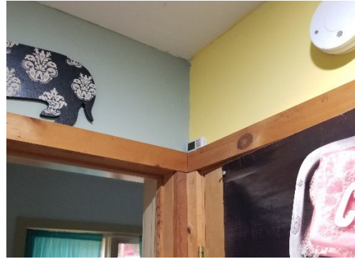
Temp/RH Sensor in First Floor Hallway
