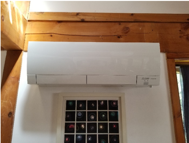
Upstairs Indoor Unit
