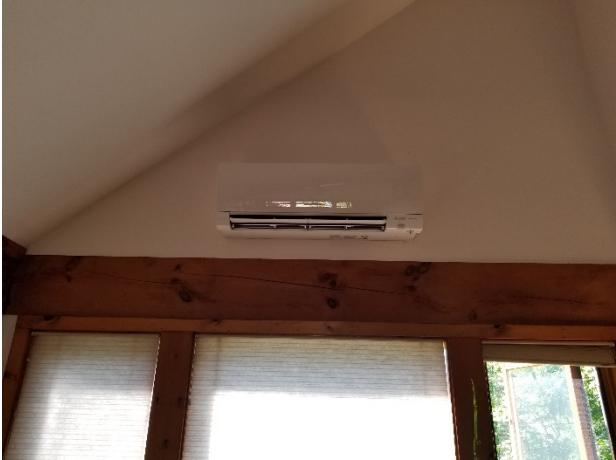
Living Room Indoor Unit
