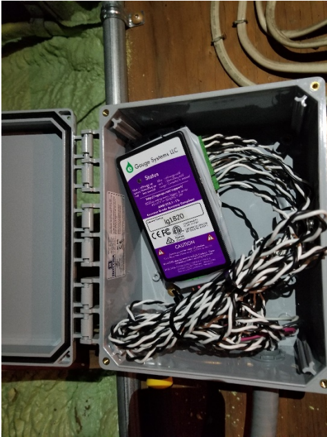
eGauge Monitoring Box
