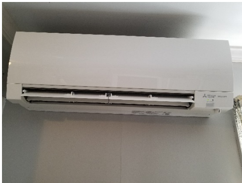
Kitchen/Dining Room Indoor Unit
