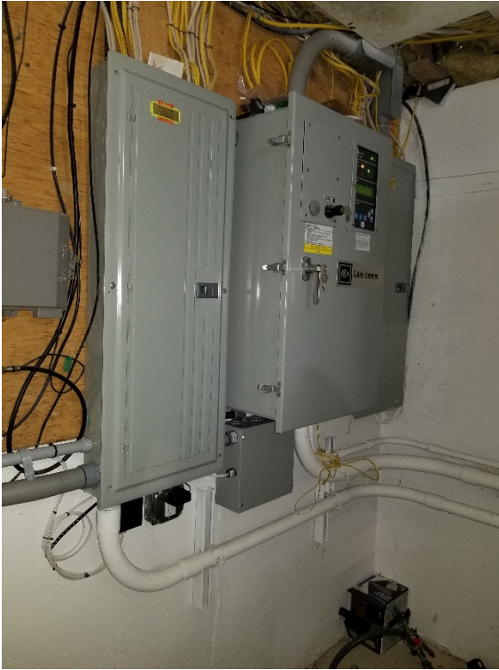
Main Electrical Panels with eGauge 36446 Enclosure
