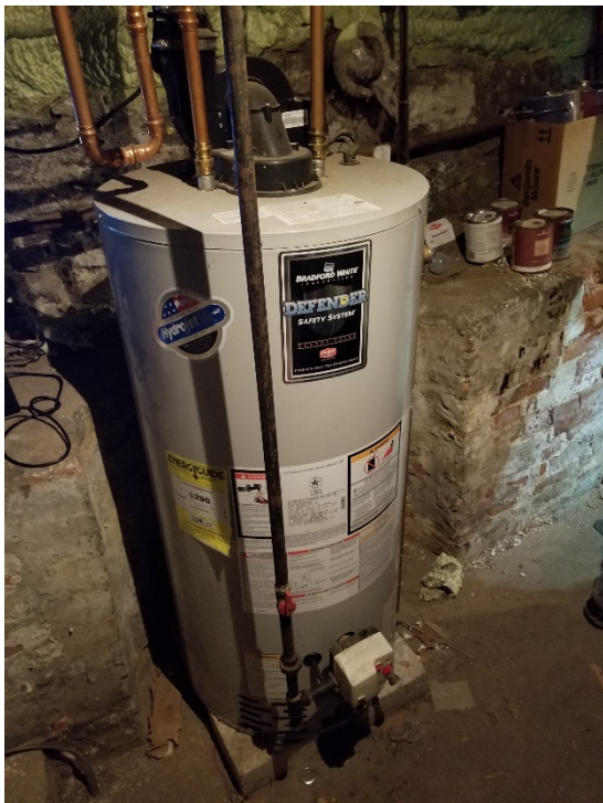
Natural Gas Storage DHW
