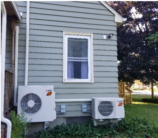
Kitchen/Dining and Master Bedroom Outdoor Units
