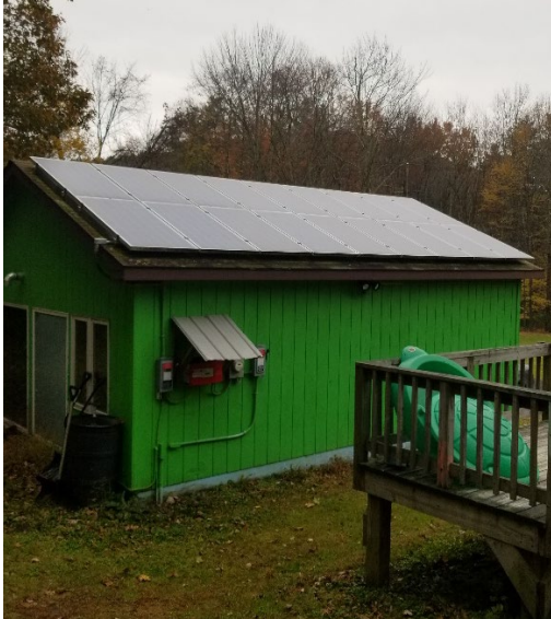
2.5 kW PV Array on Garage
