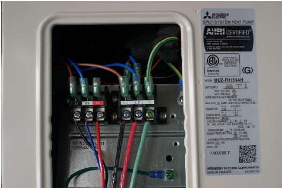
Outdoor Unit Wiring and Nameplate
