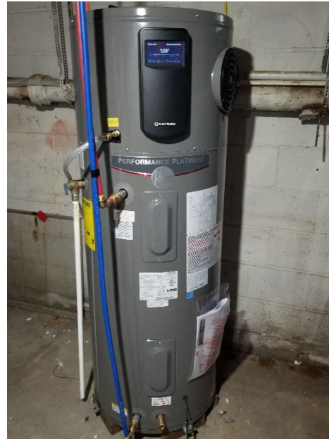
Electric Heat Pump DHW
