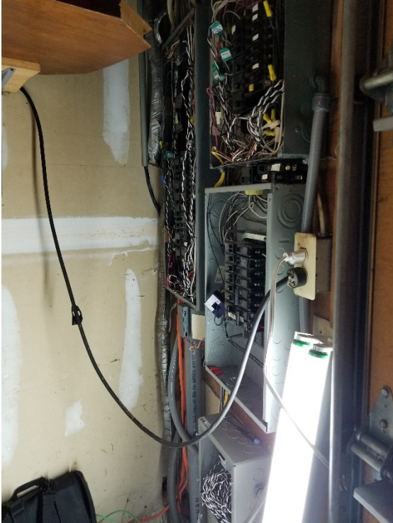
Main Electrical and Secondary Panels with eGauge and CTs
