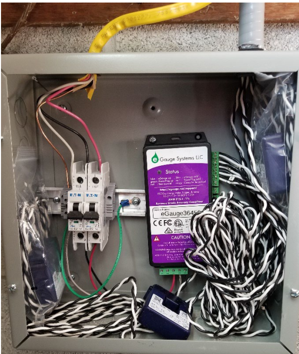
Data Logger Enclosure with eGauge
