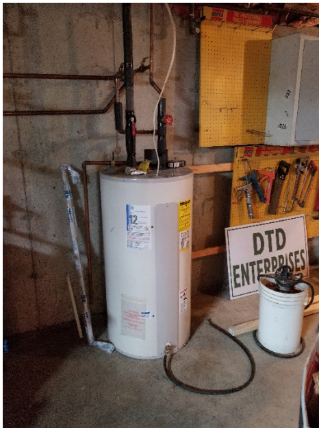
Electric Storage DHW
