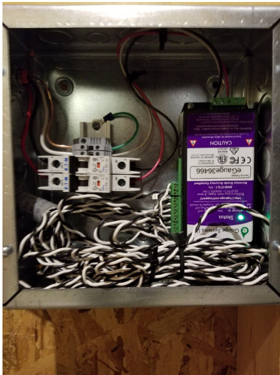
Data Logger Enclosure with eGauge
