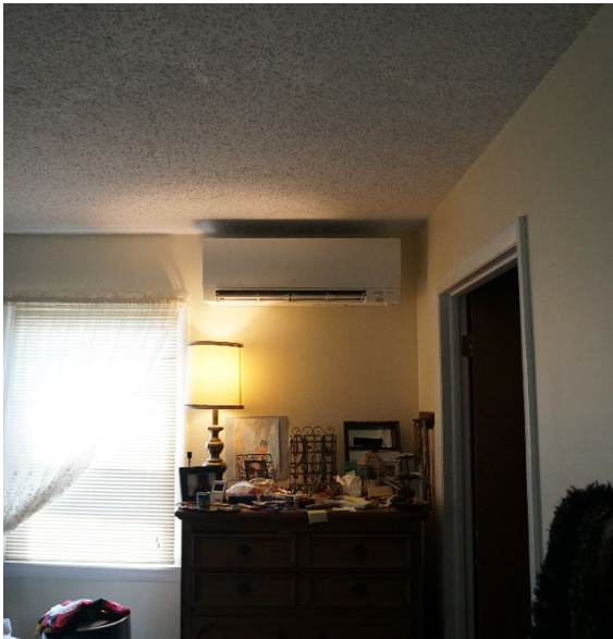
Master Bedroom Indoor Unit
