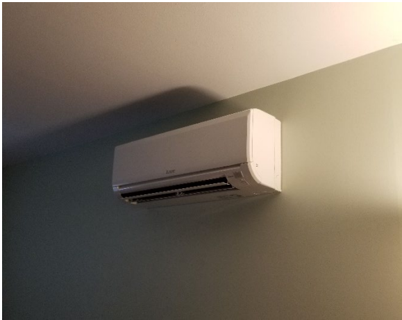
Master Bedroom Indoor Unit
