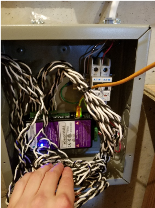
eGauge Monitoring Box
