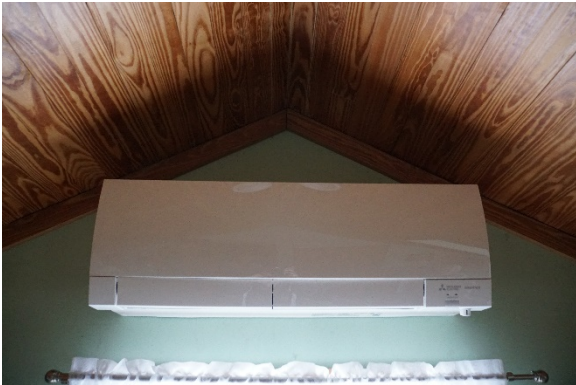
Master Bedroom Indoor Unit
