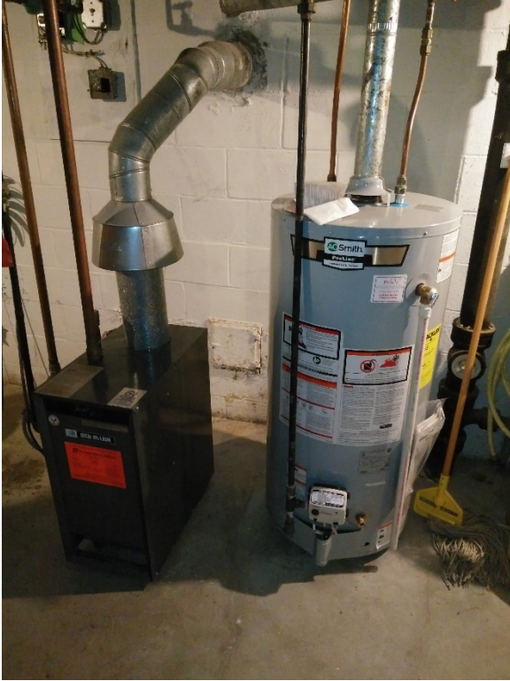
Boiler (L) and gas DHW heater (R)
