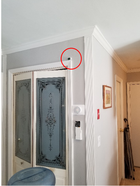
Temp Sensor in Kitchen
