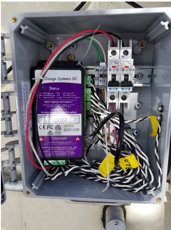
Data Logger Enclosure with eGauge
