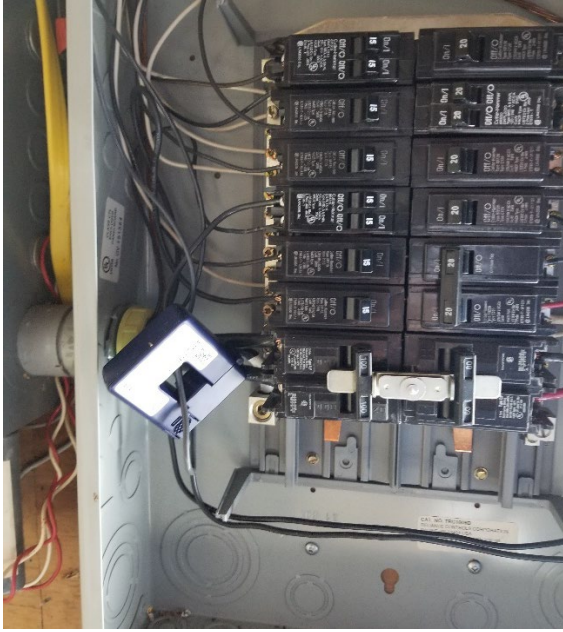
Secondary Electrical Panel
