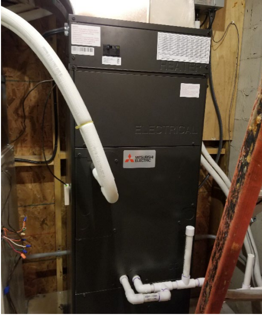
Air Handler Located in Basement
