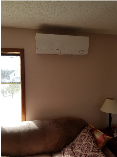
Upstairs Indoor Unit
