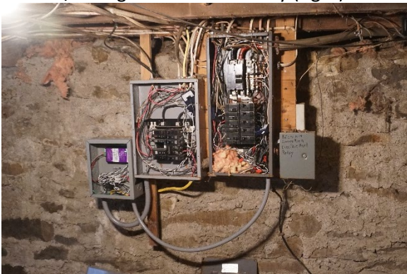
Installed CTs and eGauge Panel
