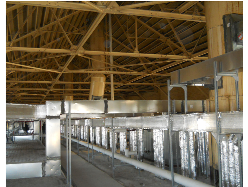
Clean Mechanical Space
