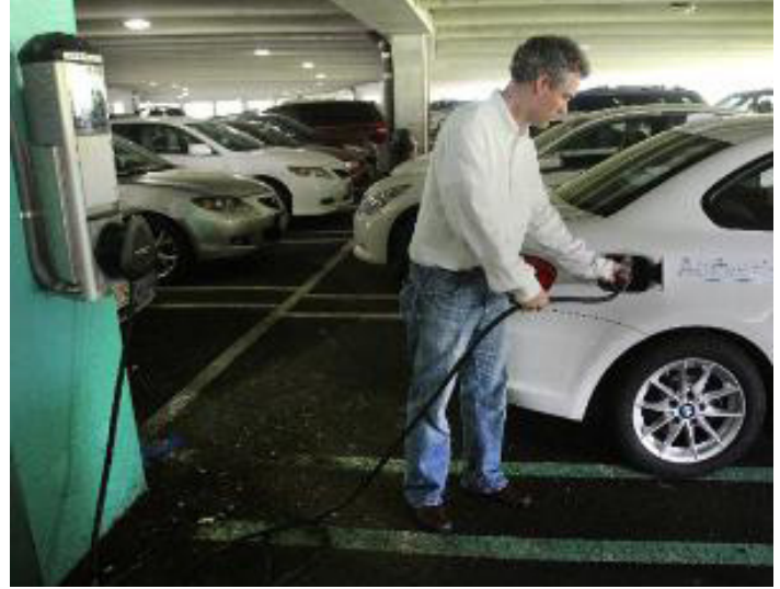
IMAGE 4. PARAMUS, NJ BY MOUNTING THE EVSE ON AN EXISTING POST BETWEEN SPACES, PARKING SPACE SIZES ARE MAINTAINED AND WHEEL STOPS OR BOLLARDS DO NOT NEED TO BE INSTALLED
