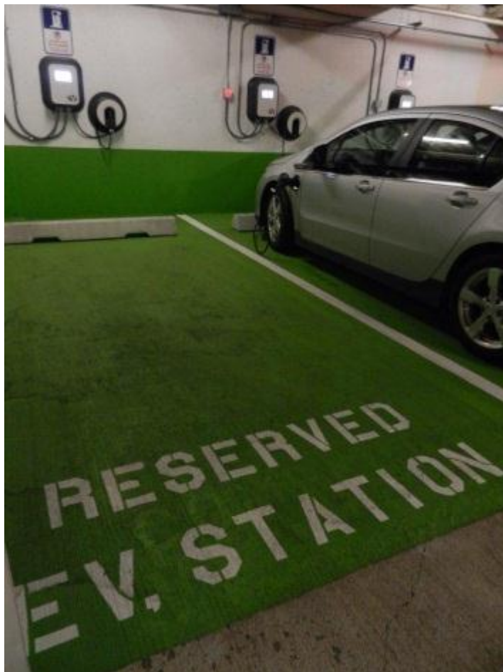
EV charging station marked with paint
