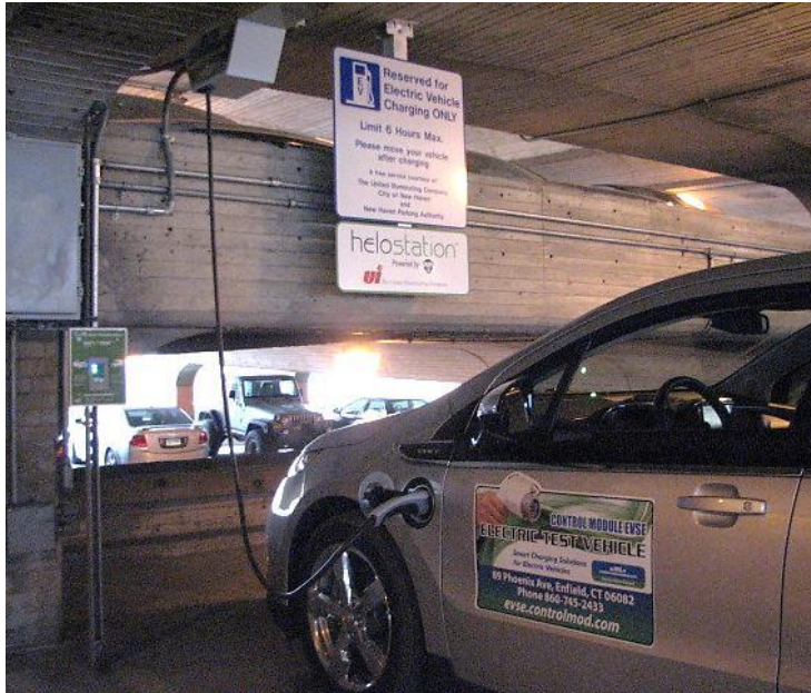
Level 2 EV charging cable automatically lowers from ceiling (photo courtesy of EVSE Ltd.)
