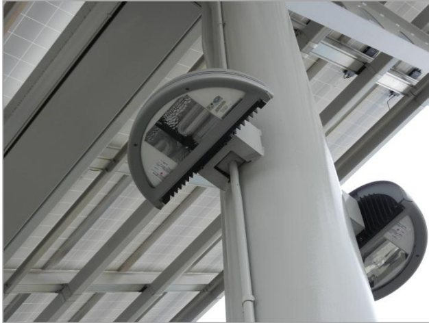
Lighting installed above EV charging station
