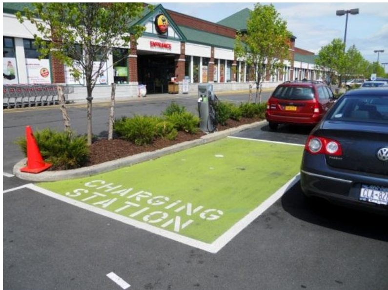
EV supply equipment can reach two parking stalls (Photo courtesy of Capital District Transportation Committee)
