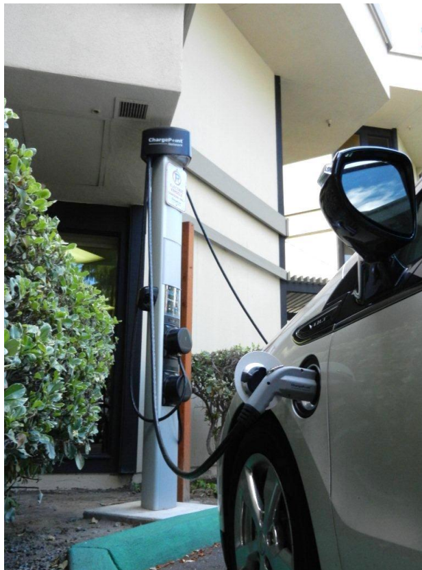
Level 2 EV charging cable retracts
