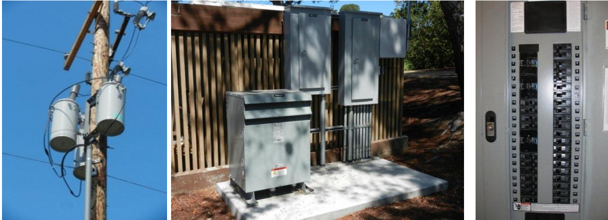
From left to right: (1) pole-mounted transformers; (2) surface-mounted transformer and electrical panels; (3) circuit breakers in electrical panel
