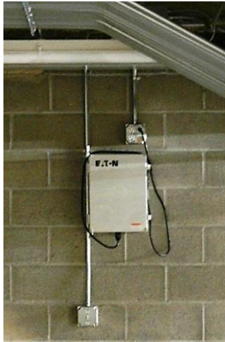
Cellular modem for group of EV charging stations
