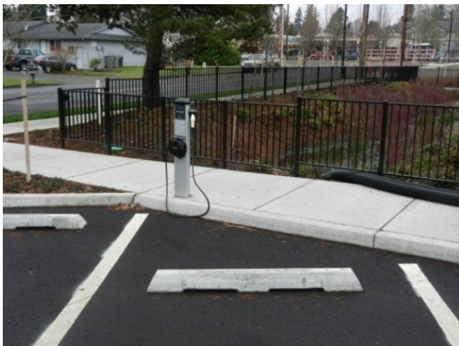
Pedestal-mounted EV supply equipment well-located at angle parking
