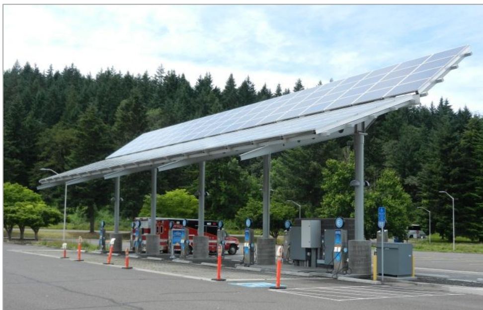
Solar canopy with EV supply equipment
