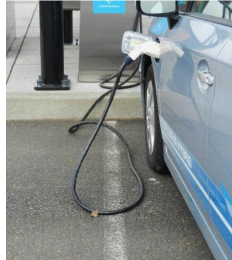
Cables can create tripping hazard
