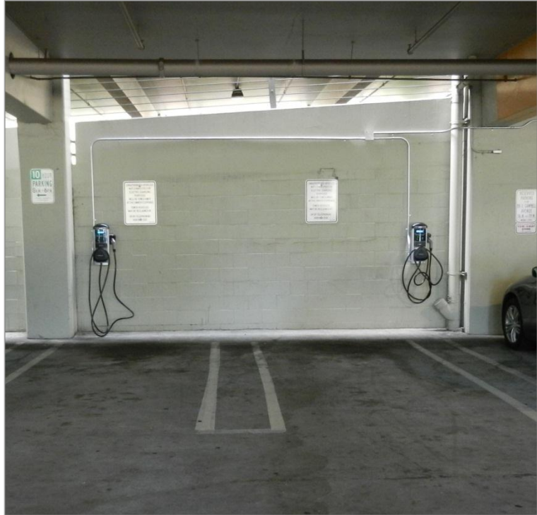
This installation inset between posts includes no wheel stops or bollards
