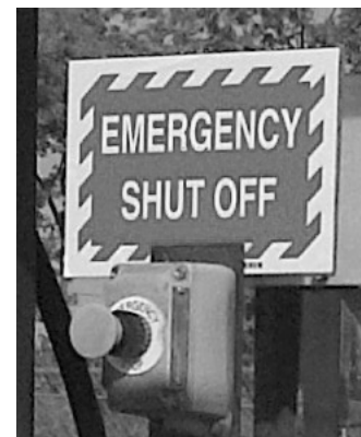
Figure 14. Emergency shut-off buttons for compressed natural gas maintenance facilities and fueling infrastructure
